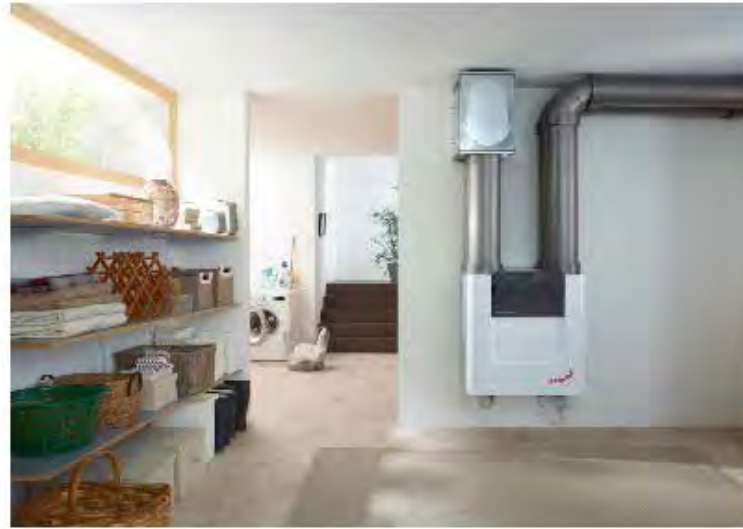
Indoor Ventilation & Heat Recovery
